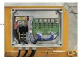
▶ Electric Control System
